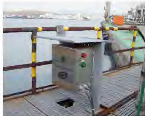
Figure 3 – Terminal/Pier Oil-Sensor & Alarm
