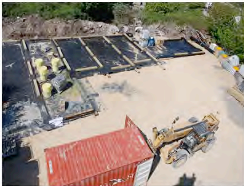
Fig. 4 Bunded areas especially created by Braemar Howells Ltd. for dealing with the HNS from the containers
