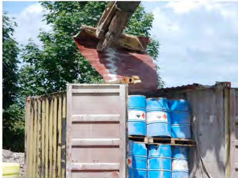
Fig. 7 Lid of the container being removed to access the damaged drums
